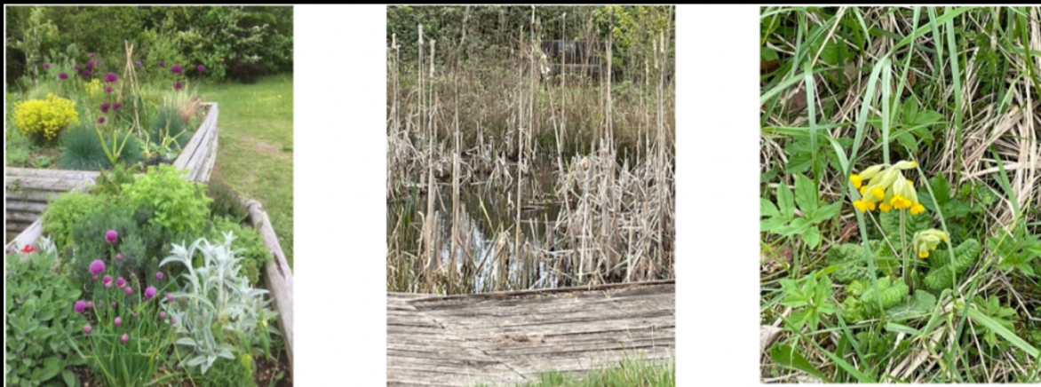
Sensory beds and pond viewing platform showing repairs needed. A pretty little cowslip.
